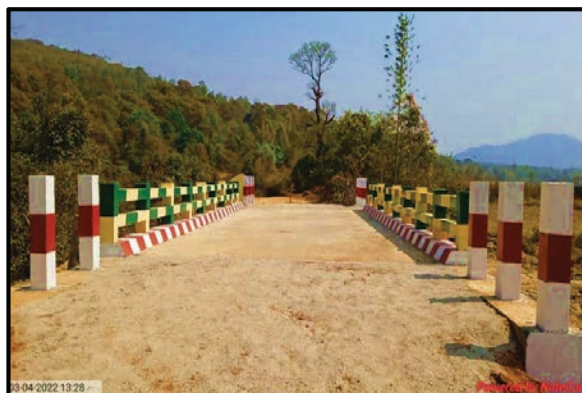
Construction of 40 feet concrete bridge on Kaungsan-Wannaug village tract in Lelchar Township
