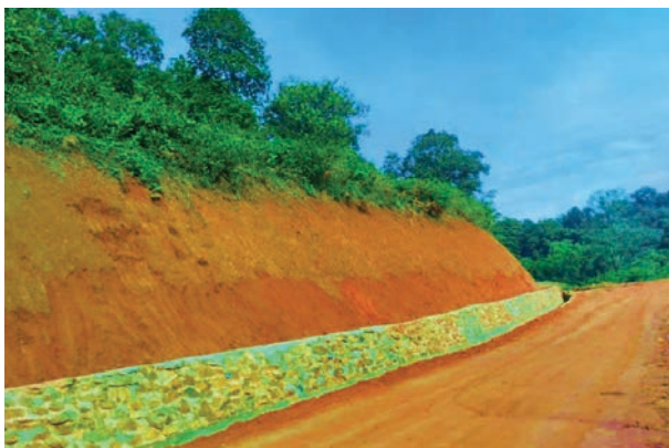
Construction 3000 feet of stone pitching drain on the road of 4 miles army camp Gyikelwe-Naboke-Susii in Chipwi Township
