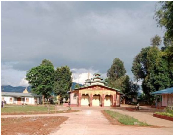
Paving 1350 feet concrete road among 1700 feet in Soon loon monastery entrance road, Loilen Township, Southern Part of Shan State
