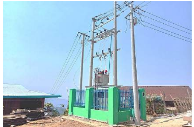
Installing 2 Transformers in Hwaysan village, Sahaung village tractLoilien Township, Southern Part of Shan State
