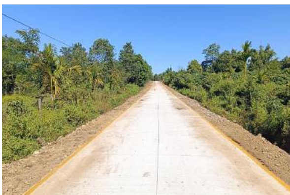
Paving concrete ( consist extension of earth road) in Naung Chaing village access road in Waingmaw Township, Kachin State
