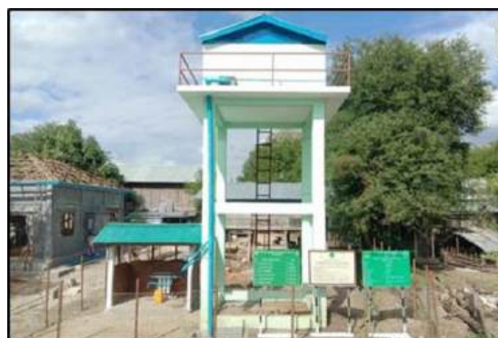
Installing Pipe line and Purified water system at Kha Laing Village, Min Hla Township, Magway Region
