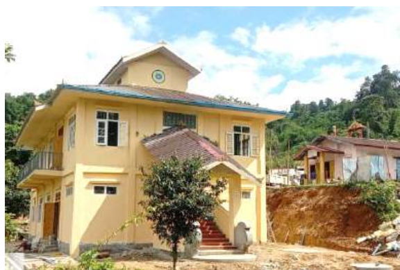
Construction of 53 x 30x 24 feet RC two- storeyed religious building (Central Monetary), Chipwi Township, Kachin State
