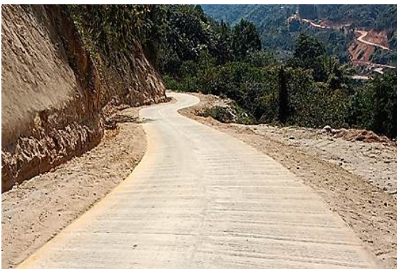
Paving 1 miles concrete road among 19 miles in Susee- Taung Thone lone-Matlivkaw road from 4 miles Camp among 52 miles in Chipwi –Sotlaw, Chipwi Township, Kachin State
