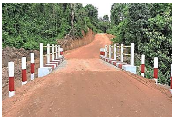
Construction of 20 feet concrete bridge on Kyuhti- Narma (1) road in Maingsatt Township, Eastern Part of Shan State
