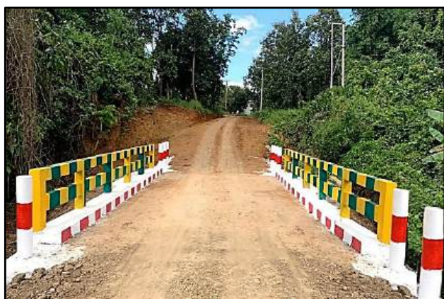
Construction of 25 feet concrete bridge on Pain Chit – Wamkone village access road in Pain Chit village tract, Loikaw Township, Kayah State
