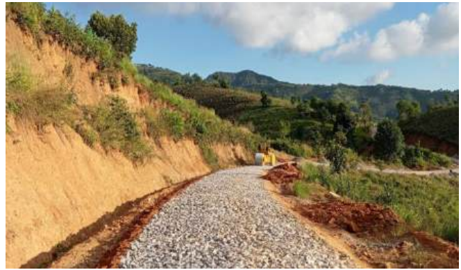
Paving 1 miles gravel road on the 6/5 miles remaining road in Taryaw-Yarthit-Nyaingkone-Shweminphone pagoda-Alaeywar-Sawetaw-Taungpae road from No (8) Wart in Kalaw Township, Southern Part of Shan State
