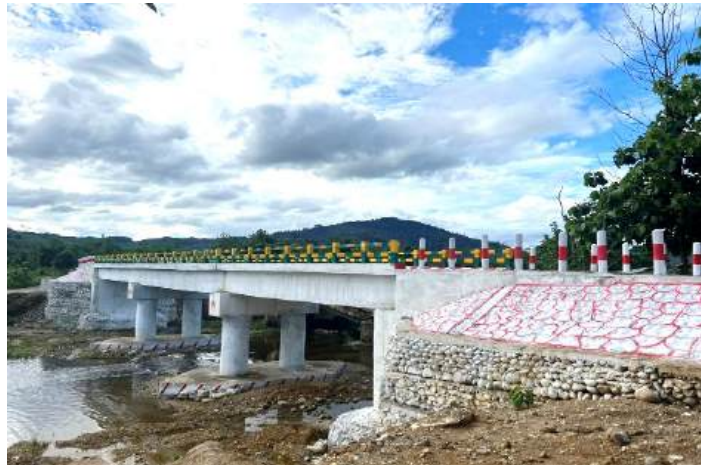
Construction of 125 feet concrete bridge on Inhukha creek in Lawaryan Village , Waingmaw Township, Kachin State
