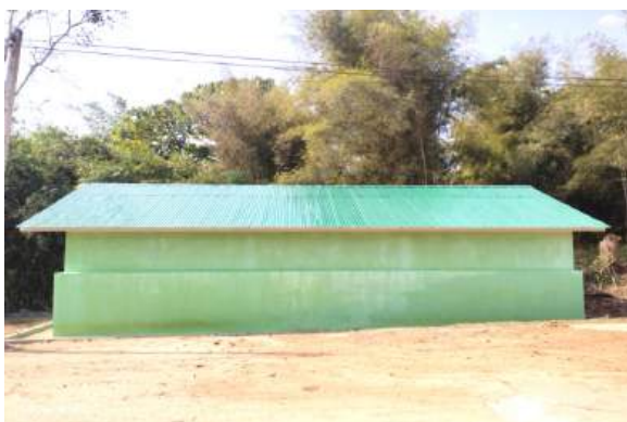
Construction of 2000 gallon water storage tank to supply water in Parla, Makhay, Maiklont, Phweyhai and Maankhan villages, Tarchileik Township, Eastern Part of Shan State
