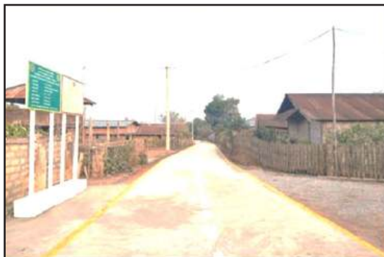
Paving concrete road in Man Kaung Village, Tantyan Township, Northern Part of Shan State
