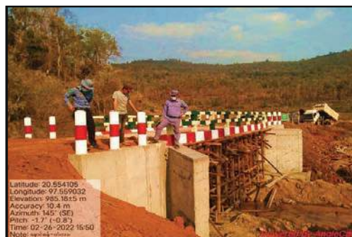
Construction 35 feet concrete bridge on (7/4) miles Namtsan- Naungbo road in Namtsan Township
