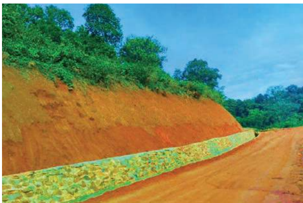
Construction 3000 feet of stone pitching drain on the road of 4 miles army camp Gyikelwe-Nabokey-Susii in Chipwi Township
