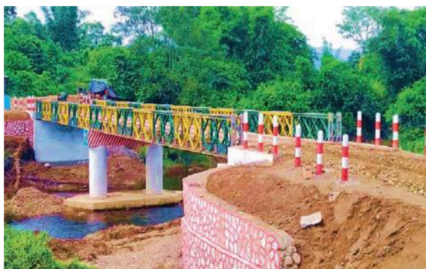
Construction of 130 feet bailey bridge on the access road of Lantaung-Naungkhing village in Putao Township
