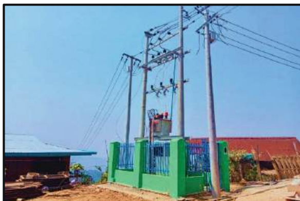
Installing of transformers in Hwaysan village, Sahaung village tract in Loilem Township
