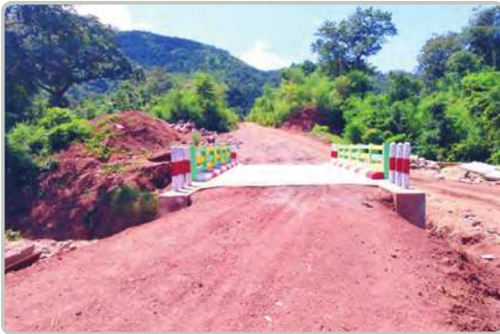
(5) feet of Box Culvert on (2/0) miles of Teemar-Tanakine-Lonehtan road in Kutkhaing Township
