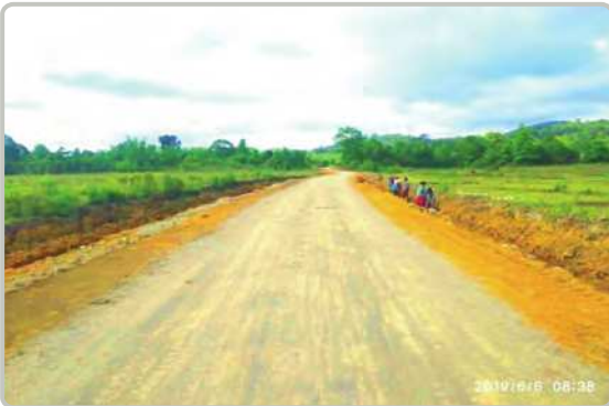
(1/4) miles of gravel road from Putao to Namhtwalkhu road in Putao Township
