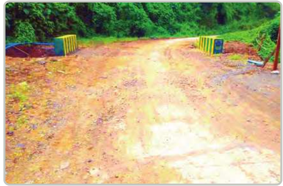
(5) feet of Box Culvert on (2/0) miles of concrete road at Khaingkam-Painpi in Tedim Township
