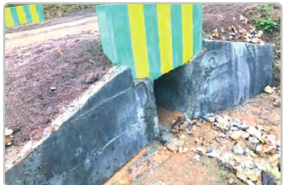
(3) feet of concrete pipe culvert on (2/0) miles of gravel road at Lwekan-Naunghan-Namrain in Kutkhaing Township
