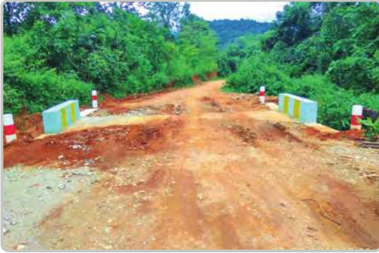
(4) feet of Box Culvert on (8/3) miles of Yarapra-Yosapra-Kroko access road in Hpruso Township
