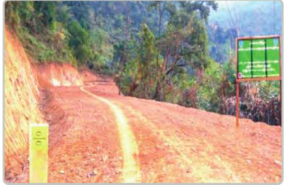
(1/0) mile of earth road from Swammeyan to Inseyan road in Putao Township
